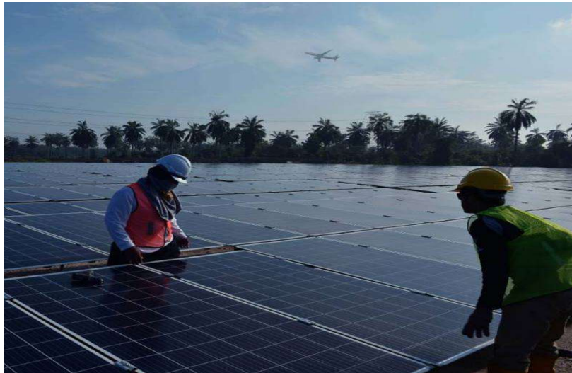
Figure 4.1: TNB Large Scale Solar (LSS) at Sepang
